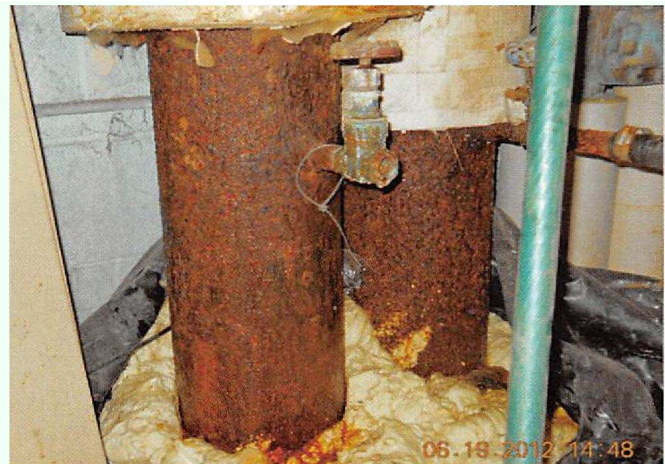
NIGHTMARE AMATEUR INSTALLATION Interior Hot-Water and Chilled Water Supply and Return Lines with Partial Do It Yourself (DIY) Spray-Can Insulation (Expanding Foam Contained Using an Oversized Trash Bag)
